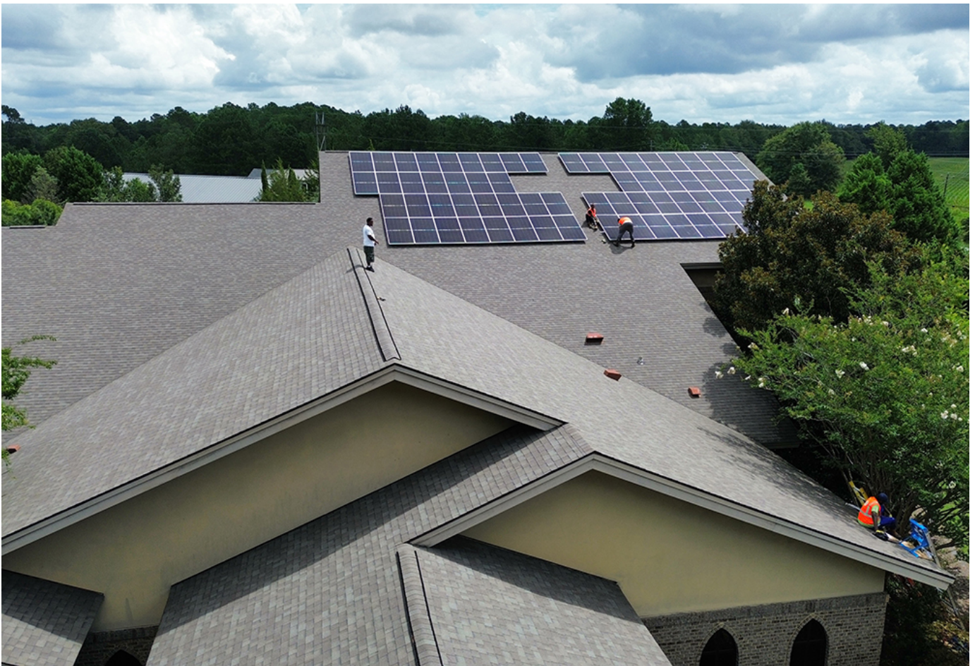
A solar installation is pictured at Trinity Episcopal Church in Statesboro, Georgia, on July 25, 2024. (Courtesy of Sunpath Solar and Georgia Interfaith Power and Light)
