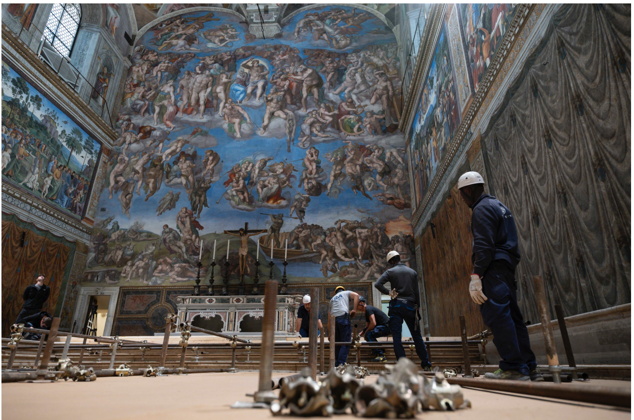
PHOTO SLIDE SHOW: In preparation for the conclave to elect a new pope, workers build platforms over a protective covering on the marble floor of the
