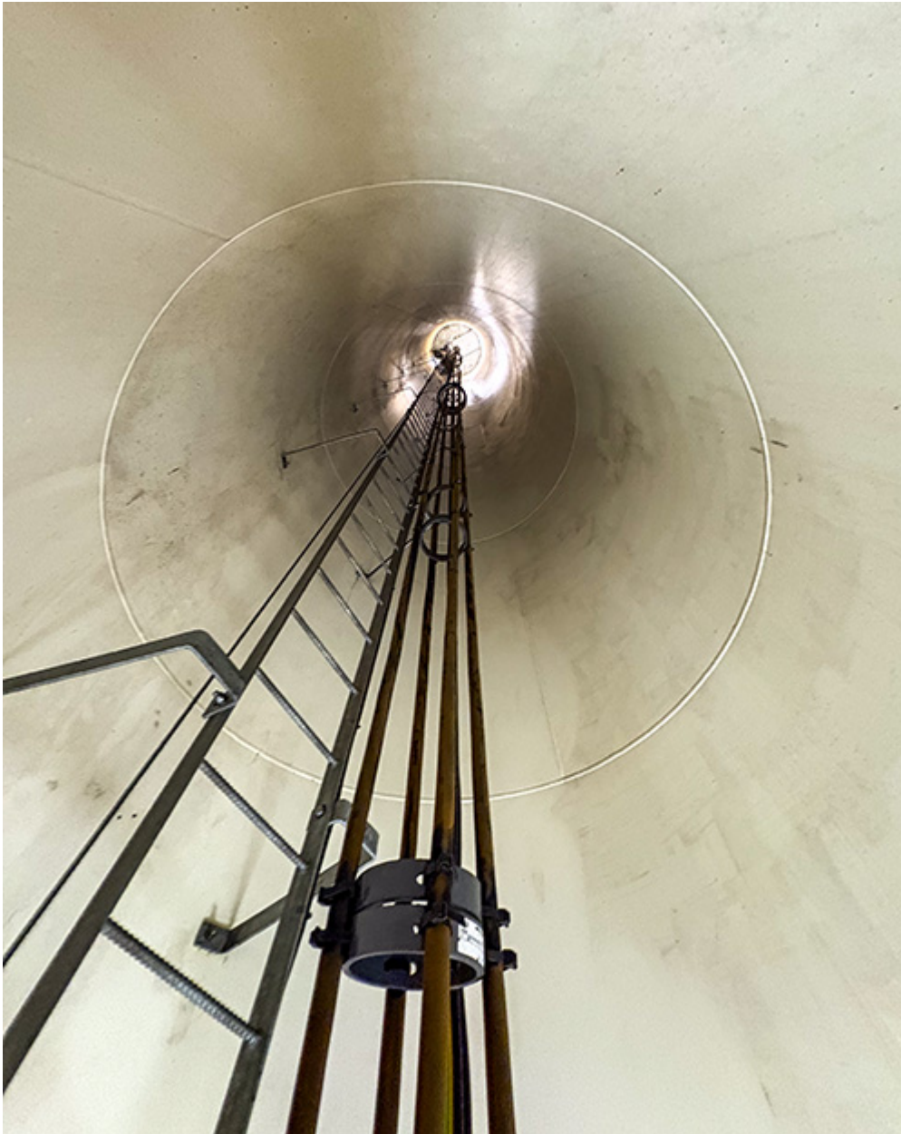
Inside the Portsmouth Abbey wind turbine, June 17, 2026 (NCR photo/Camillo Barone)
